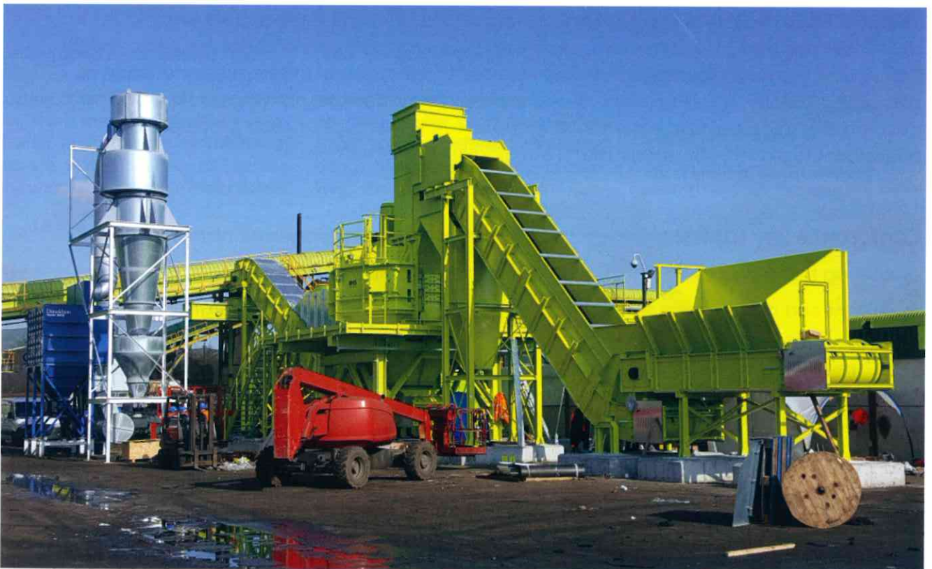
The recycling plant in the UK for processing automotive shredder residue (ASR) and electric and electronic scrap (WEEE) was still under construction here. It was planned and implemented by BHS-Sonthofen (©CMüller)
