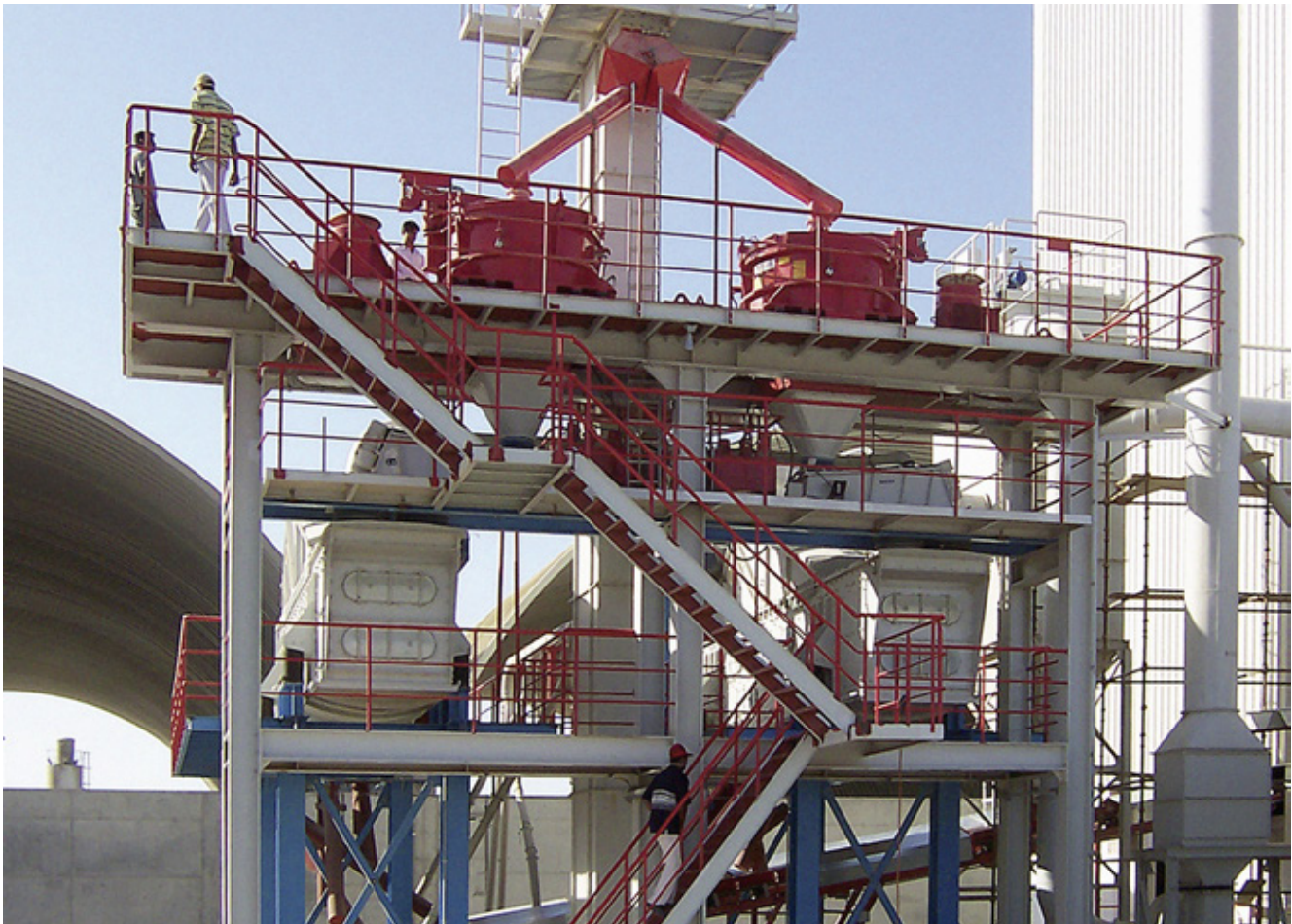
Use of two RPM 1513 rotor impact mills in a dry-mortar plant in the United Arab Emirates (UAE)
